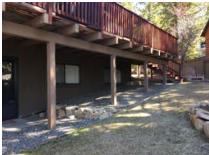
Figure 5: The under-deck area should be considered in the noncombustible zone, including managed vegetation and removing combustible materials. (Photo: Shearman Builders)
